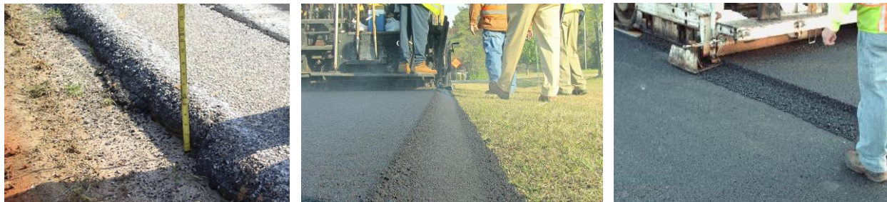
Examples of pavement edge drop off (left, FHWA, 2017), Safety Edge (center, Carlson Paving, 2017), and notched wedge joint (right, Willow Designs, 2017) treatments.
