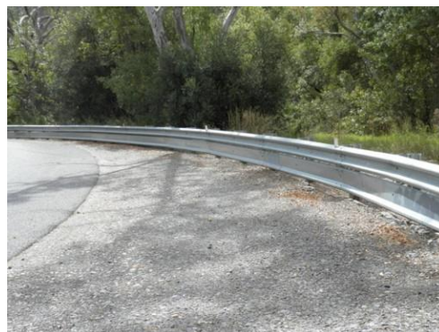
Examples of guardrail continuous protection systems (Department of Planning, Transport, and Infrastructure, 2017).
